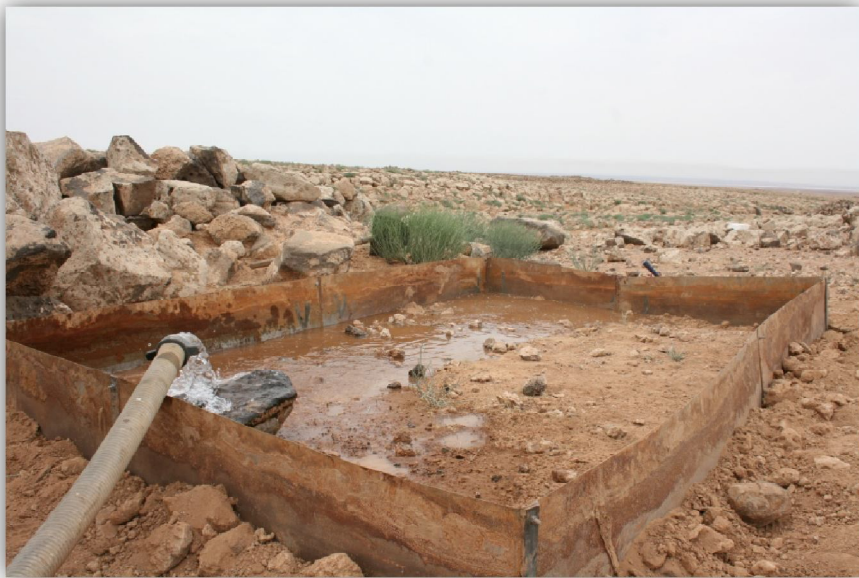
Photos 20, 21: Installation and implementation of second BIT in Mafraq Safawi Western site.
