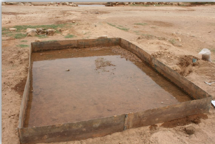
Photos 32m 33 and 34: Installation and implementation of BIT in Wadi Dhuleil site.
