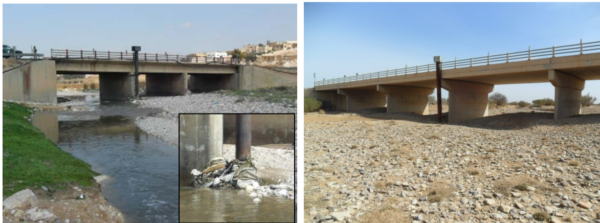
Fig. 31: left) AL0063 Zaqqa, Sukhne Station: rubbish accumulation around slotted steel pipe and station is not situated in the main flow channel; right) F0023 Wadi Butum Station: very uneven cross-section, likely to change with strong flow events. (Pictures taken by A. Steinel, 2012).
