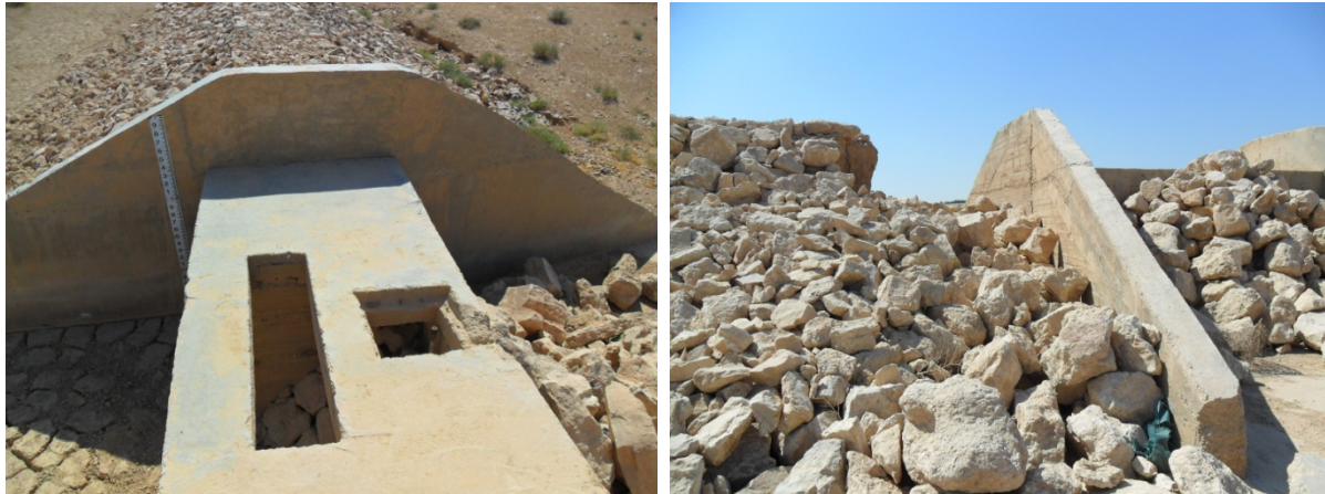
Fig. 14: Wadi Madoneh: left) dam M2: metal parts from gabions and manhole were stolen and release pipe opening/closing mechanism blocked with large stone, right) dam M1: damage to dam due to the use of material not adhering to the specifications (Picture taken by A. Steinel in 2011).
